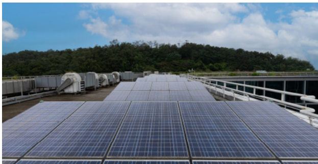
Solar Power System
