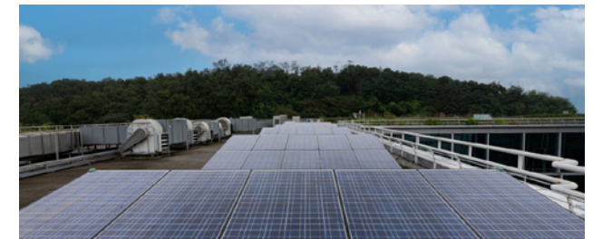
Solar panels at the Pangyo business site
